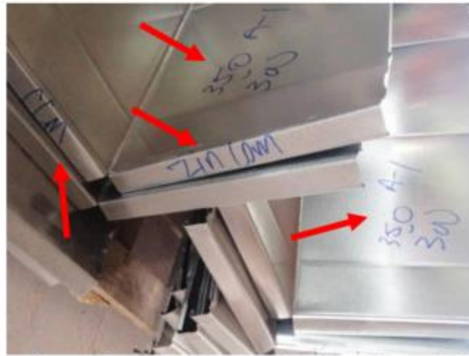
Image 39: Marker ink on duct surface that need to be cleaned.
