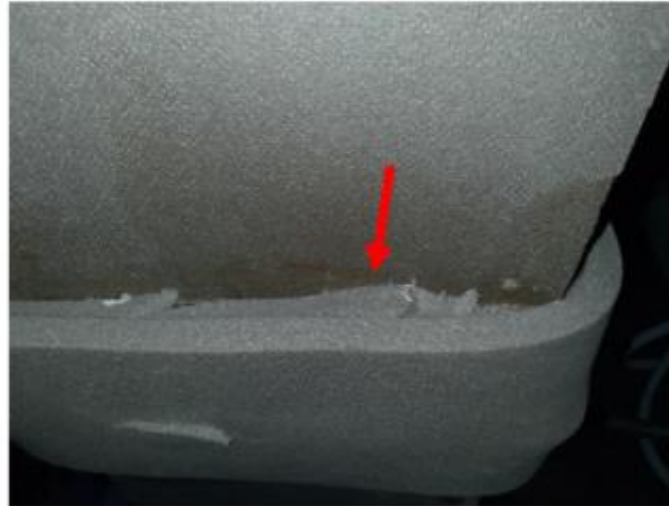
Image 72: Ripped at the edge of insulation.
