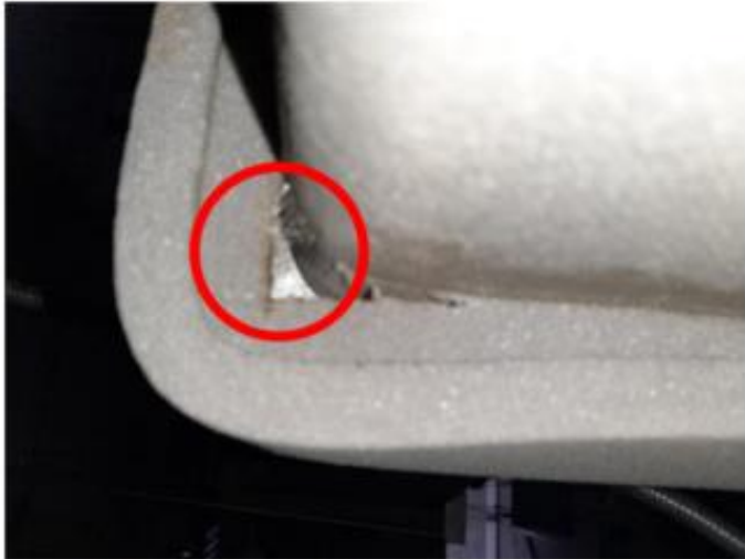
Image 71: Hole at the corner of insulation.
