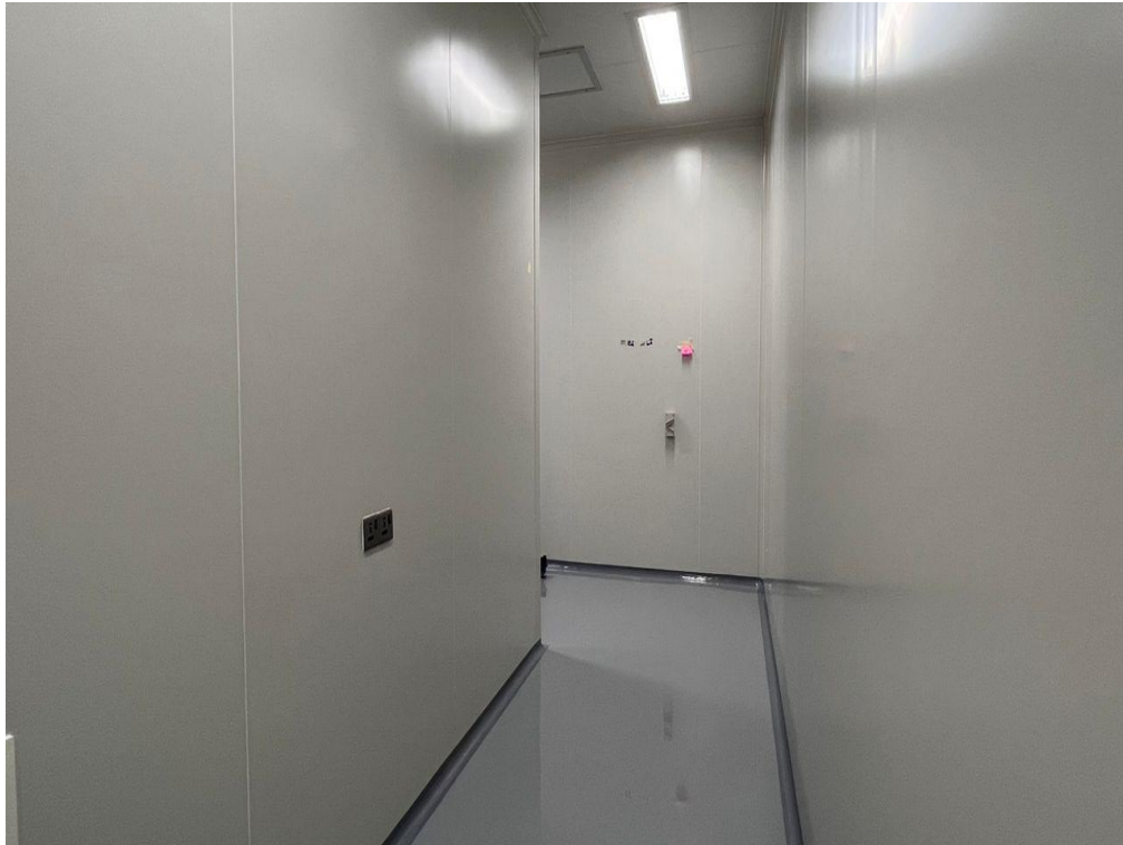
Image 25: Technical Space (View 1)
