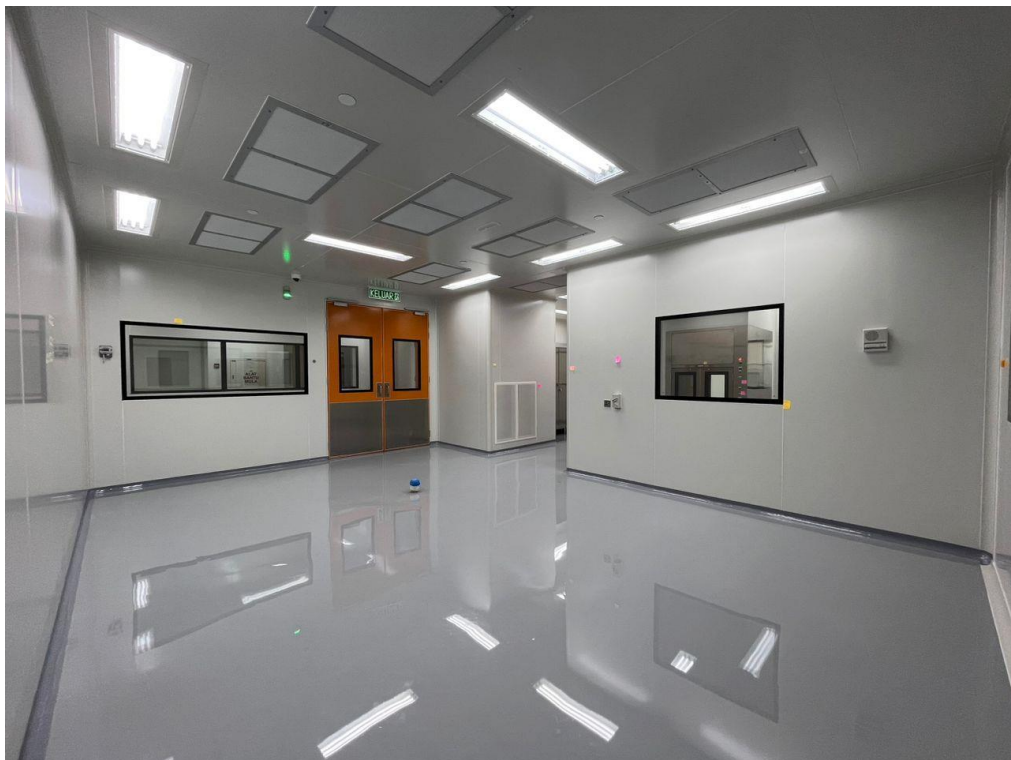
Image 14: Component Preparation Room (View 2)
