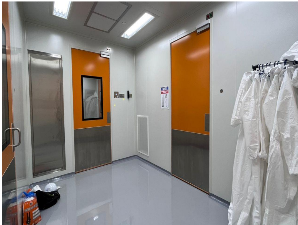
Image 51: Personnel Airlock In / Out (View 1)
