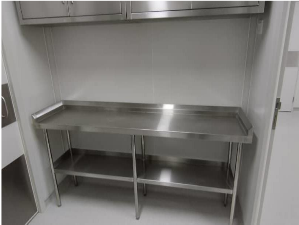
Image 9: Packing & Autoclave Room 2 (View 2)
