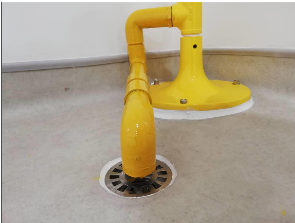
Image 22: Nurse Station Site Condition (View 3)
