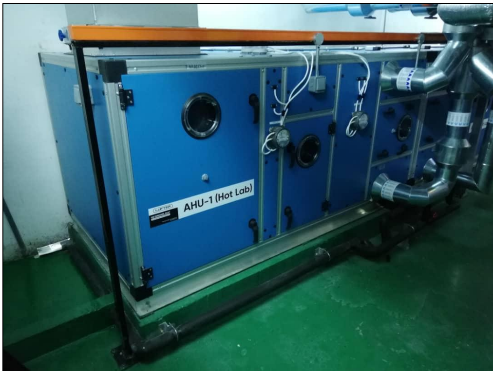
Image 32: New AHU Room for HotLab Internal Site Condition (View 1)
