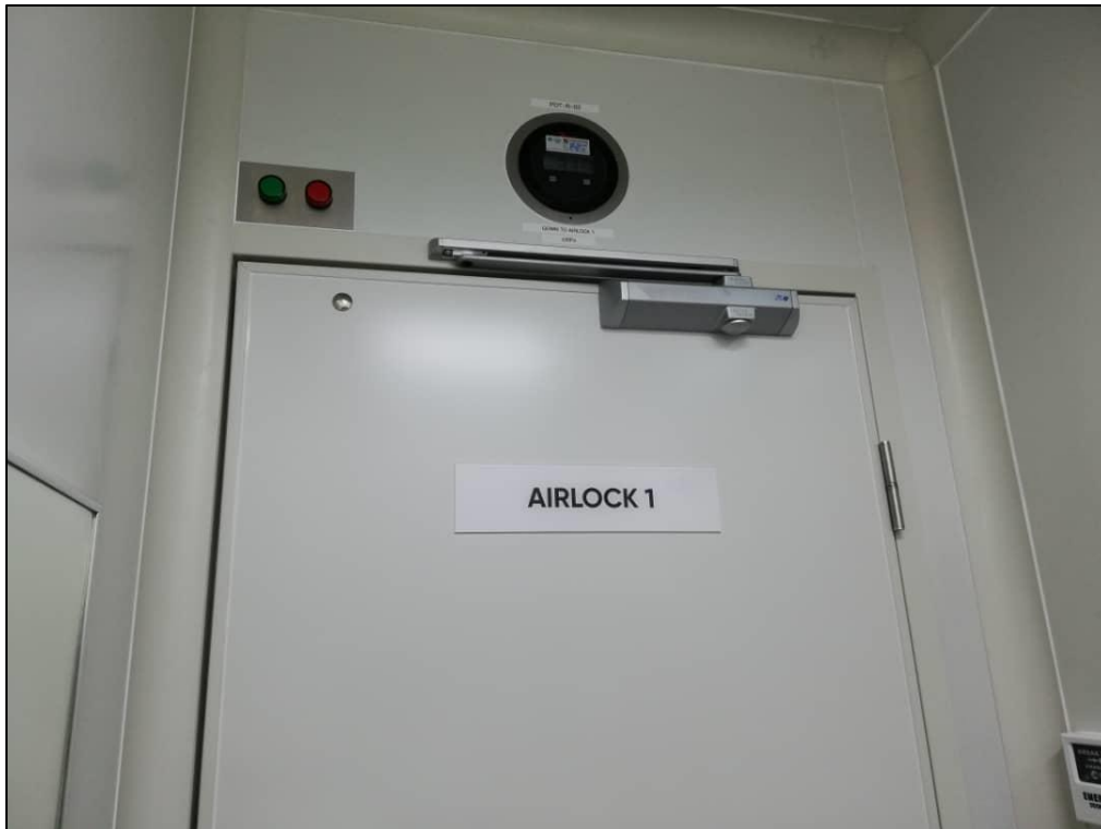
Image 10: Gown Room Internal Site Condition
