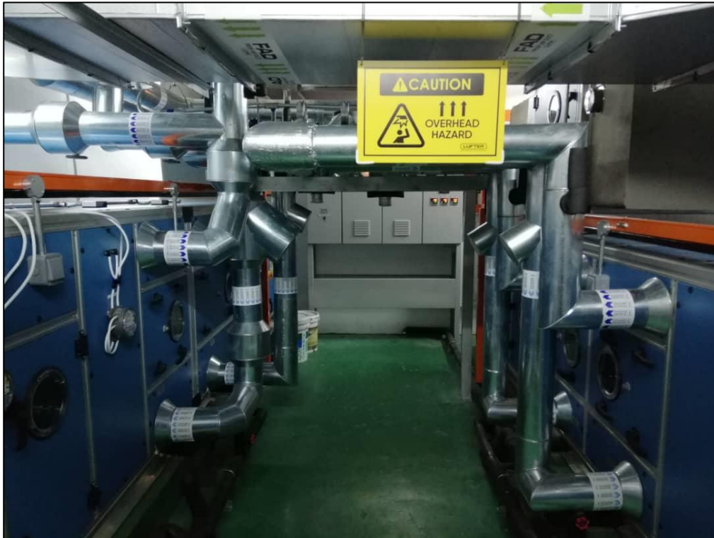
Image 33: New AHU Room for HotLab Internal Site Condition (View 2)
